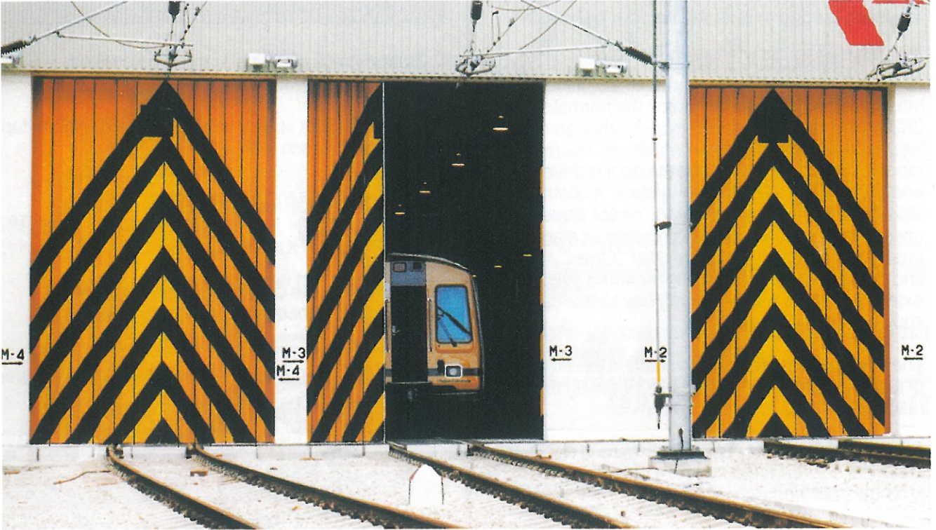
FOLDING SHUTTER INSTALLED FOR K.C.R.C. WITH LEADING EDGES CUT OUT FOR CABLES PASS THROUGH
